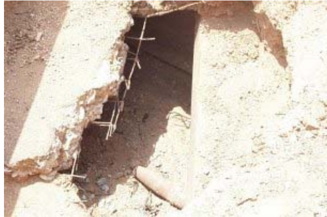
[The photograph above shows] where the accident happened.]
